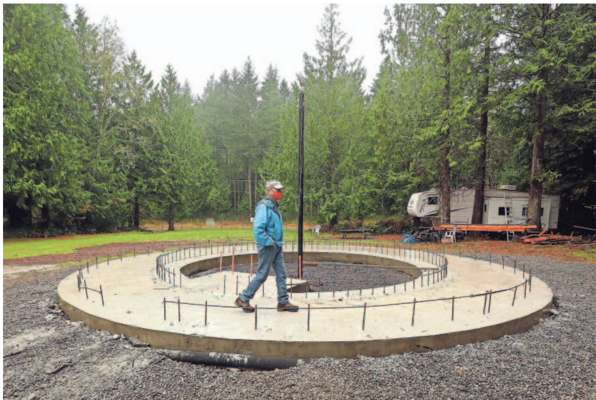
Tom Rogers, of Poulsbo, walks around the concrete base of what will become a peace pagoda at Ground Zero Center for Nonviolent Action in Poulsbo. MEEGAN M. REID/KITSAP SUN
